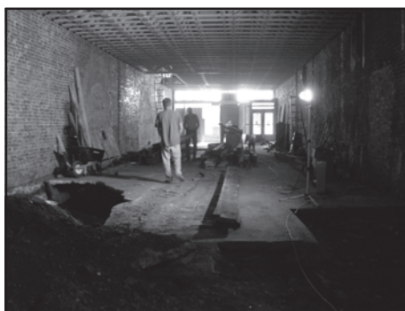
Digging inside in low lighting was slow going, and the extreme heat didn't help things much.
